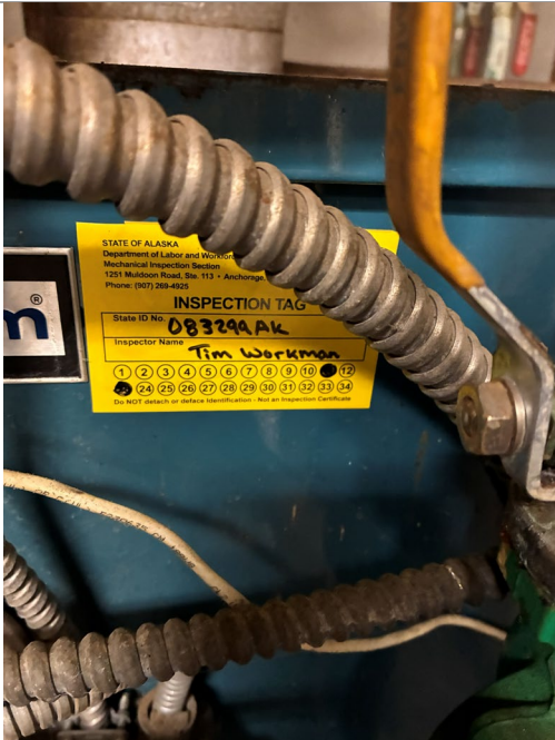
11-099C-26A: Rental (Old Clinic); The boiler was last inspected in November of 2023. It is recommended an inspection take place as soon as possible to ensure all components of the boiler are functioning as designed.
