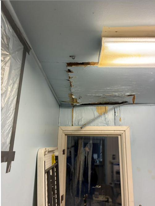
03-099C-26A: City Hall; Water has leaked through the roof, impacting insulation and weatherization inside the building, the finishes (mostly aesthetic), and potentially, the structural stability of the building. Water was also observed to have pooled in the lights at some point.
