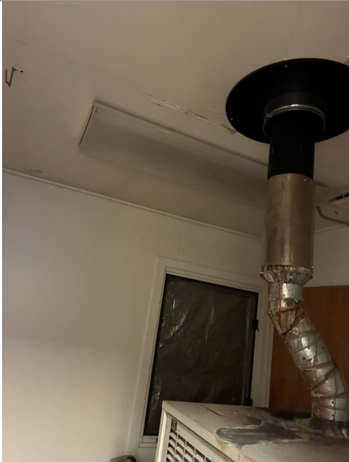
01-099C-26A: City Hall; The light did not function in the furnace room on the DMV side of the building. It is recommended to repair or replace this light so maintenance and visual checks can be safely conducted.
