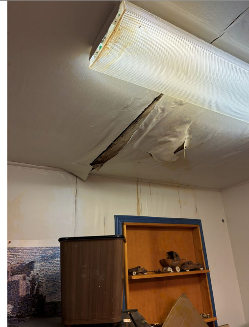
04-099C-26A: City Hall; Roof leak cont: Where water comes in contact with electrical connections, this could compromise the electrical system and result in overheating and potentially a fire. In the roof's weakened state, the structural stability is questionable for excessive snow loads. It is recommended the roof be repaired or replaced. A structural engineer should evaluate the structural stability of the entire building once the old roof is removed.
