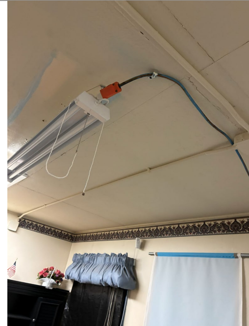
02-099C-26A: City Hall; An extension cord was used to run power to the light in the DMV office. Extension cords are for temporary use, so it is recommended power be run to the light in a fixed installation.
